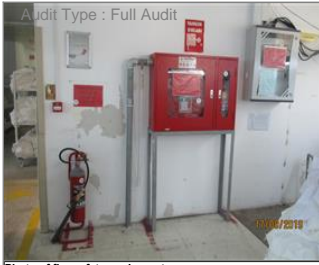
Photo of fire safety equipment FIRE EXTINGUISHER AND FIRE ALARM IN SUBCONTRACTOR COMPANY .JPG
