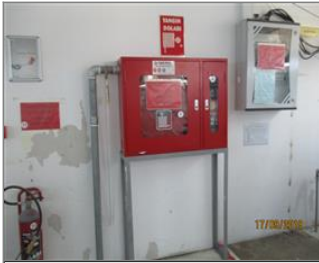
Photo of fire safety equipment FIRE HOSE AND EXTINGUISHER IN SUBCONTRACTOR COMPANY .JPG
