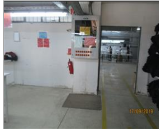
Photo of the inside of the main production hall ELECTRICAL PANNEL IN SUBCONTRACTOR COMPANY JPG
