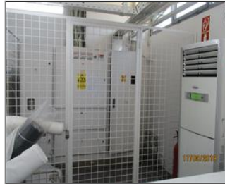
Photo of the inside of the main production hall ELECTRICAL PANNEL.JPG
