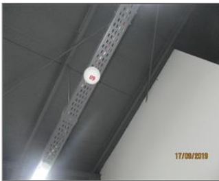
Photo of fire safety equipment SMOKE DETECTOR .JPG
